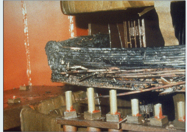
Protective systems usually can prevent damage to heavy equipment during power system upsets. However, this transformer suffered catastrophic failure during the solar storm that caused the HydroQuebec failure in 1989.
